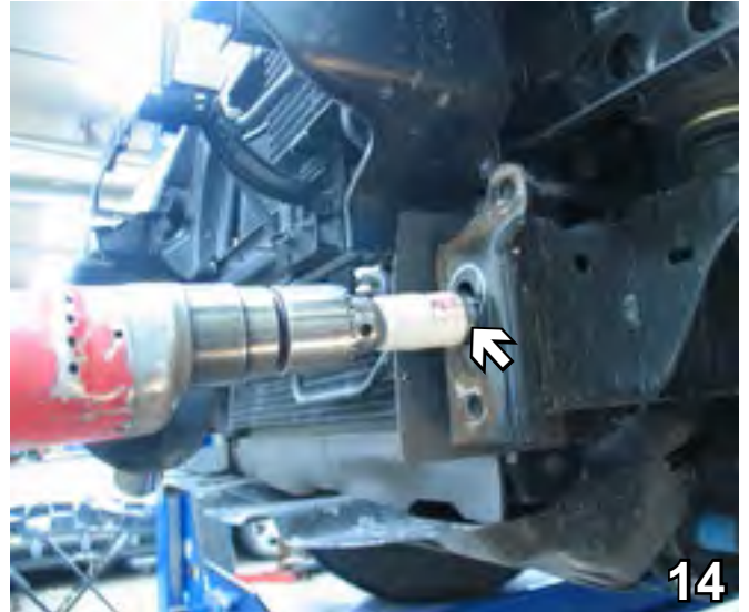
14. On the driver's side, cut a hole into the end of the frame cap connected with the upper existing hole, using the 1 1/4" hole saw, for the nut plates to go through.
