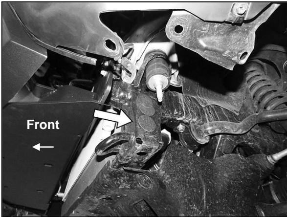
(Fig 16) Remove tape covering threaded hole in end of crossmember (arrow). Driver/left side pictured from below
