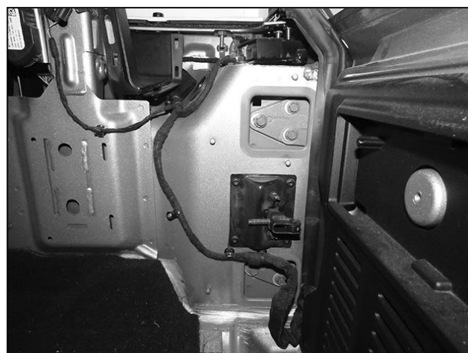
(Fig 8) Remove hardware attaching inner end of hinges to body. Slide hinges out through body
